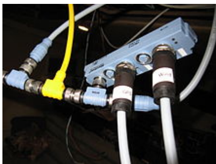
NMEA 2000 cabling using M12 connectors
